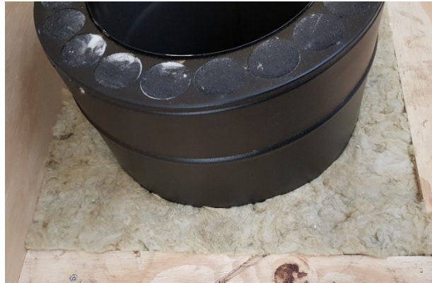
Photo 2: Insulation in first floor before it is closed by upper ceiling plate
