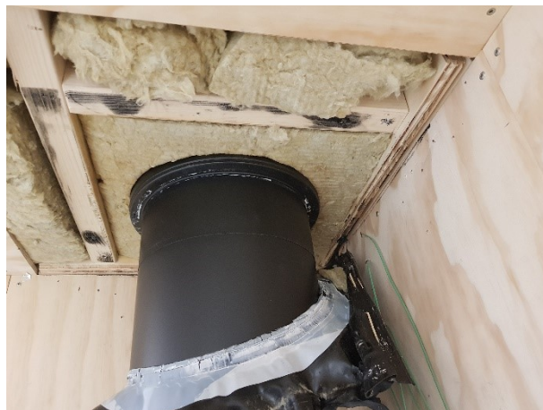
Photo 4: SabetoFLEX water vapour membrane after thermal tests. The black color on the joists is trace from the membrane.
