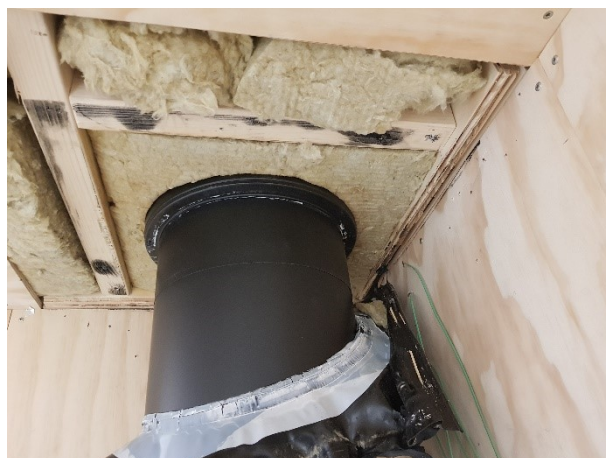
Photo 4: SabetoFLEX water vapour membrane after thermal tests. The black color on the joists is trace from the membrane.
